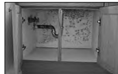
under sink mold
